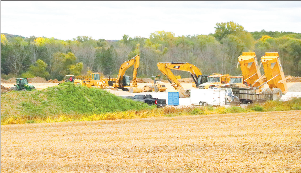
Machines and workers on-location at the construction site of the future Drexel Building Supply's Blue Door District located off Highway 28. The Village of Kewaskum annexed land from the Town of Kewaskum to accommodate the project. The project is scheduled to finish in 2025.
