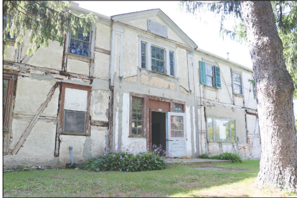
The Saxonia House at 421 Hwy H in Fillmore. MITCHELL B. KELLER PHOTOS
