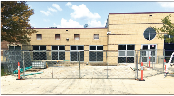
This construction project, outside Kewaskum High School, will help house a new 18-foot long cooler for the schools' food services team.
