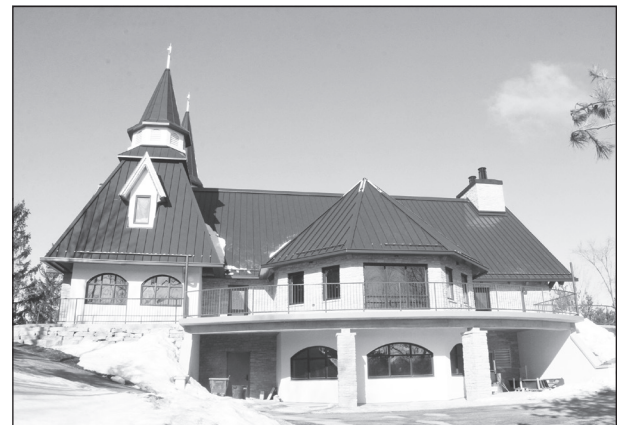
The new chapel at Camp Vista near Dundee was well underway in March 2021. The new chapel was completed in 2021 and will be dedicated in 2022. A fire in October 2018 destroyed the original chapel and construction on this new chapel started in 2020.
