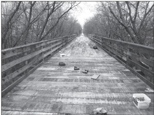
The bridge located on the Eisenbahn State Trail in Kewaskum is pictured after repairs were made.
