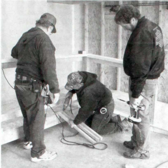
Steve Liegl, left, of Catholic Knights Insurance and Al Wollner assist Larry Bunkelman of Bunkelman Builders with a wheelchair ramp at Keith Butschlick's home in Kewaskum.
