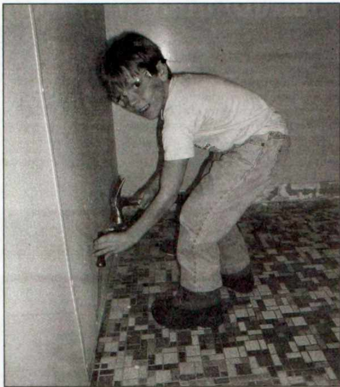
Keegan McMullen, 8, removes millboard in ladies room during a volunteer project at the town of Scott Community Center. A number of town residents and businesses pitched in to make 21st century renovations to the Community Center.
