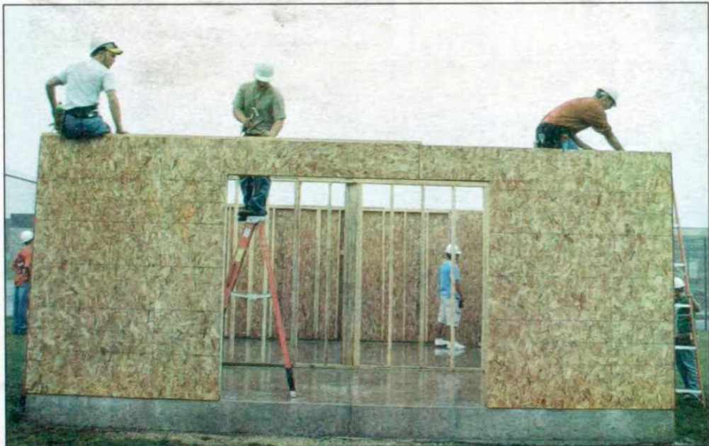
Students in Kevin Hein's Construction Skills class at Kewaskum High School have begun the process of doing the first ever "hands on construction" project at the school. They are in the process of building a shed by the tennis courts. This class works on the project daily. Watch The Statesman to see the progress of this project.
