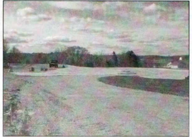
Asphalt work has temporarily been put on hold according to Parks Administrator Paul Mueller
