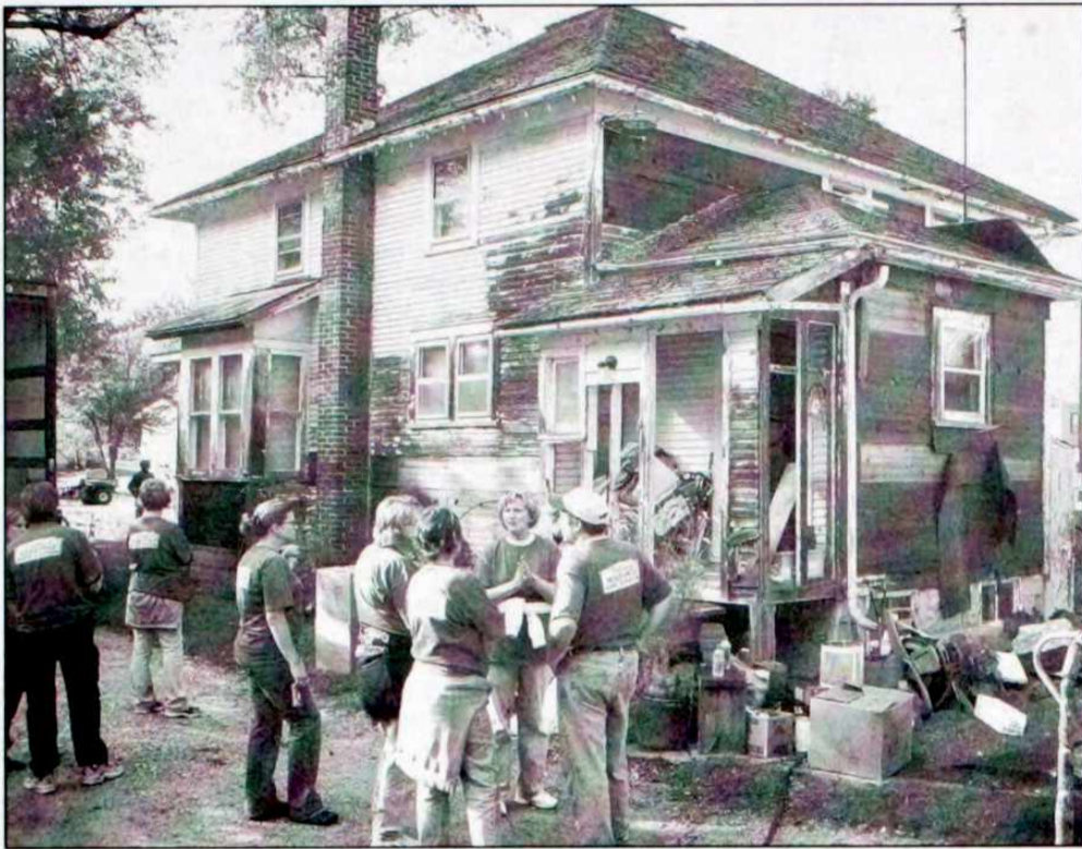
Citizen volunteers worked for hours on Saturday before demolition to remove all the Koepke family's possessions and put them into storage. Each step in the filming process involves literally hundreds of volunteers to make it move smoothly.
