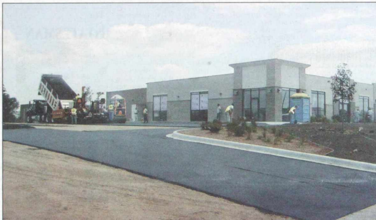
Asphalt is installed Tuesday at Kewaskum Green and Gold retail complex that has undergone extensive remodeling. Asphalt was completed Wednesday. See page three for updates on other projects within the village.
