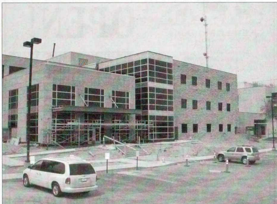
Shown above is a view of the new Washington County Justice Center that will open May 22. The justice center will be home to the Circuit Courts, Clerk of Courts and Register in Probate.
