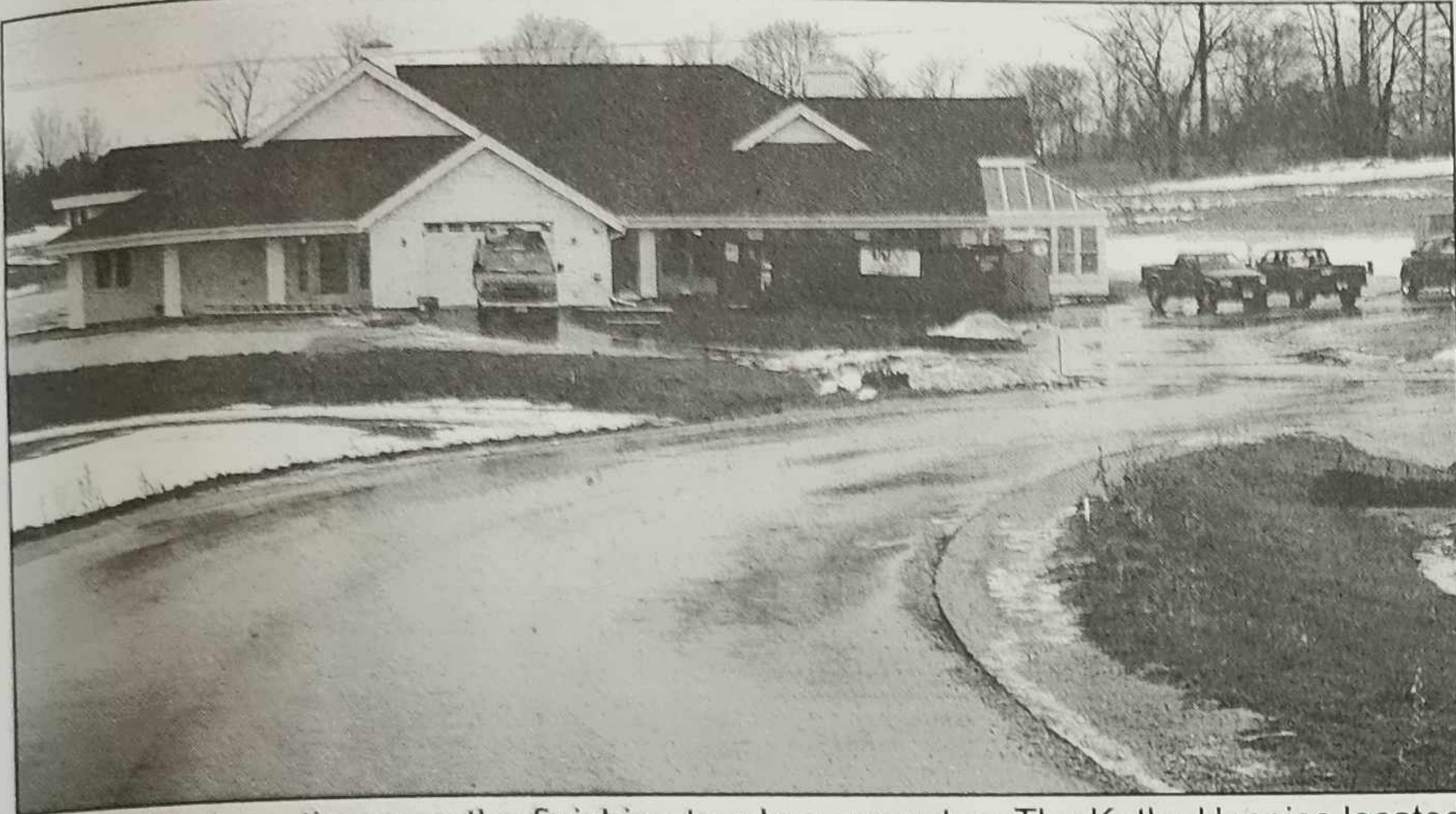
ABOVE: Work continues as the finishing touches are put on The Kathy Hospice located on the St. Joseph's Hospital campus in the Town of Polk. RIGHT: Members of SynergyHealth Foundation participate in a groundbreaking ceremony in April 2005.
