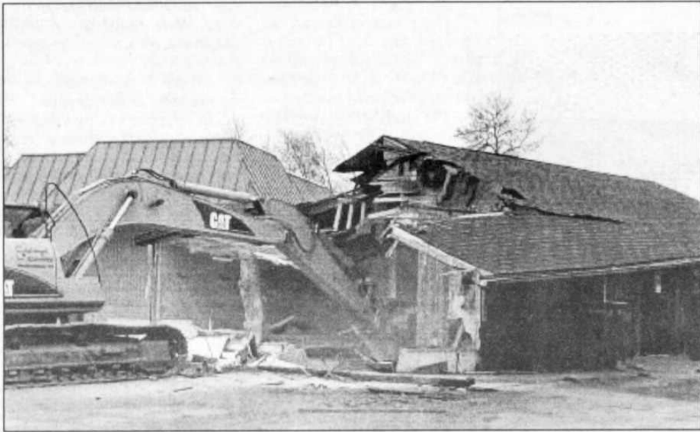
Spielvogel Excavating of Sheboygan demolished the former Marshall's Convenience Center on Thursday, March 31. The building was taken down with an hour and a half.
