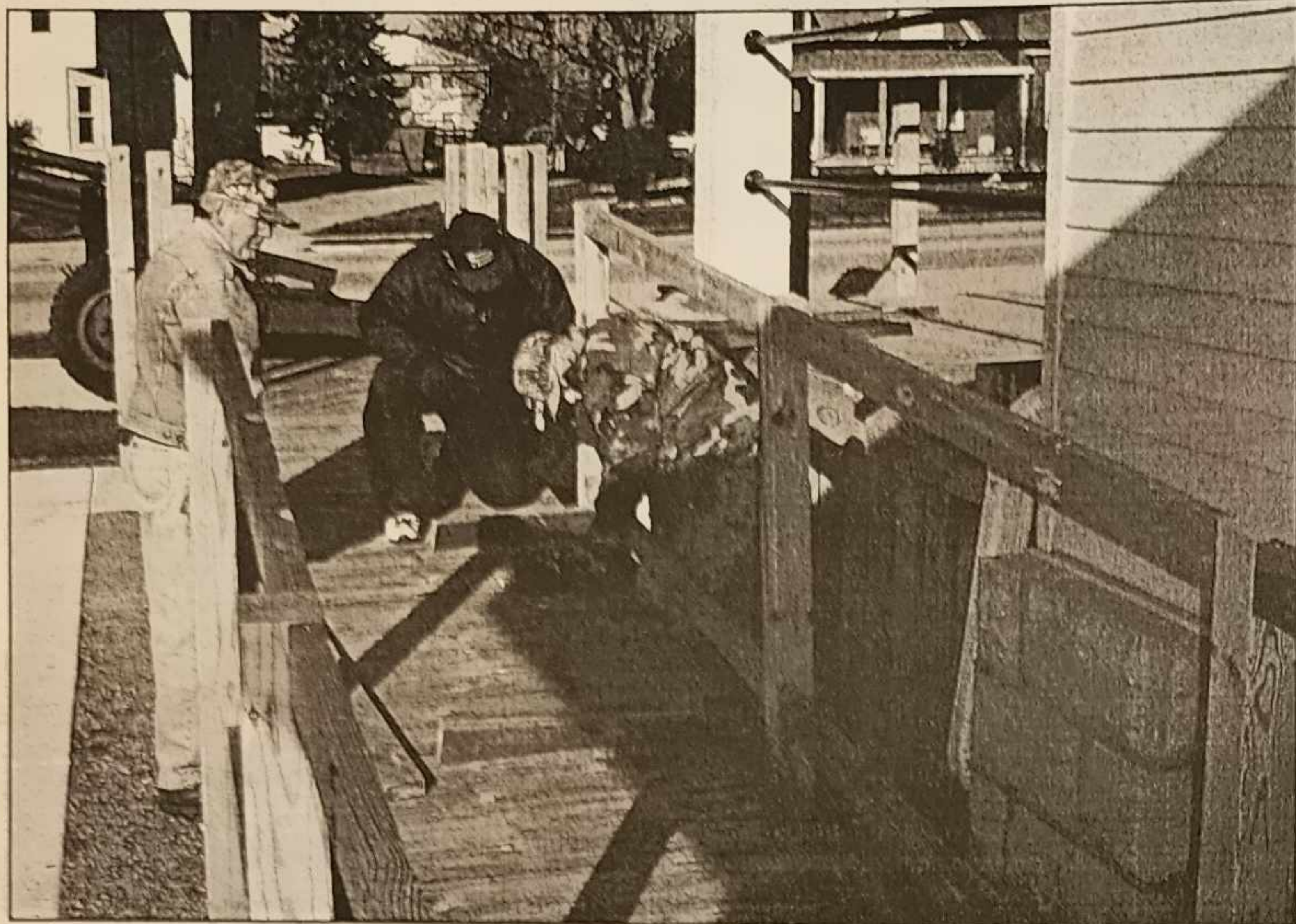
Clockwise, Roger Heberer, Al Barutha and Wayne Rimmel work on the new handicapped ramp at the legion hall.
