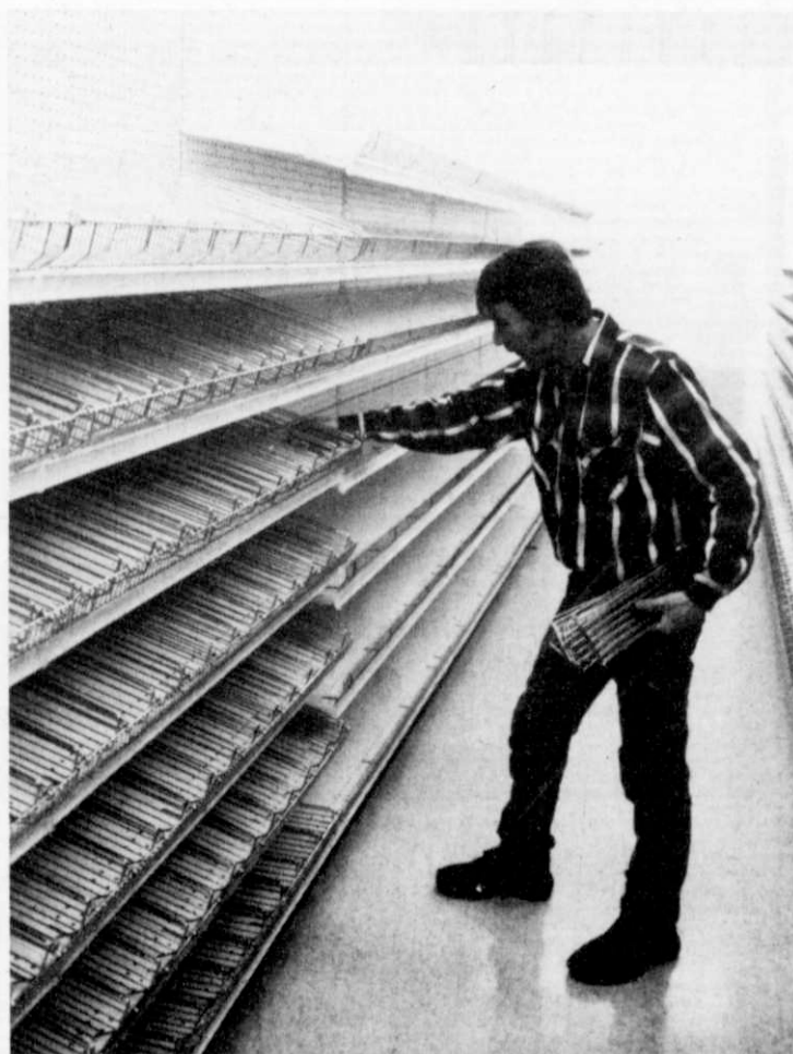
Rory Zander assembles shelving units in the newly built Tennies Ace Hardware located on Fond du Lac Avenue in Kewaskum. Store manager David Tennies stated he hopes to have the store open within the next few weeks.
