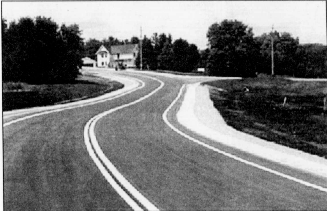
Shown above is a view looking westbound on the new Badger Road in the Town of Kewaskum that now connects with CTH H west. Traffic will start using the roadway this Friday weather permitting.
