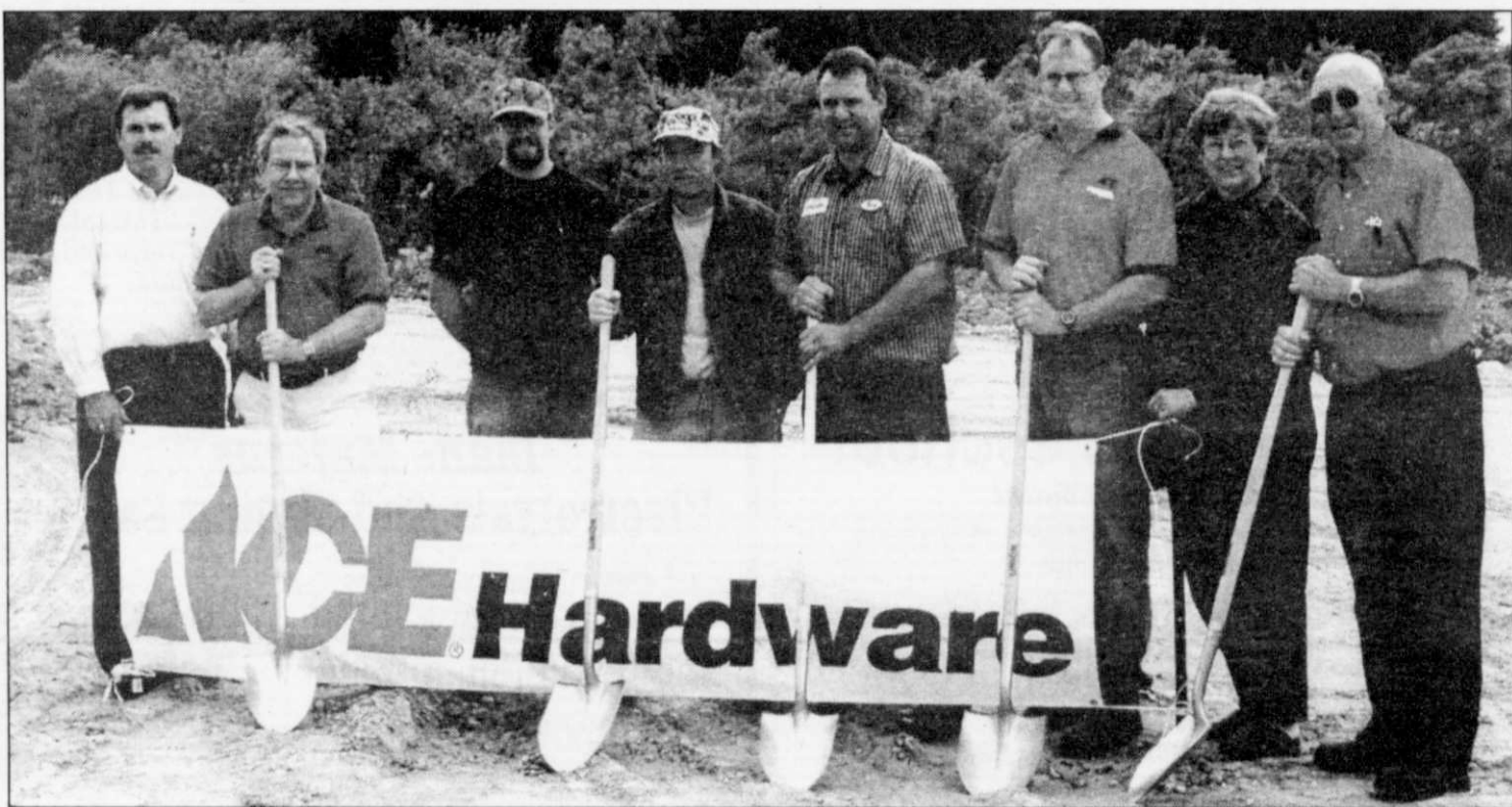
Participating in groundbreaking for Tennies Ace Hardware being built on Fond du Lac Avenue in Kewaskum were left to right, Frank Butler, Ace Corporation Midwest Division; Darryl Graff, Ace Retail Business Manager; Doede Construction Representative; Dave Doede, general contractor; Terry Tennies, David Tennies, Sue Tennies and Herb Tennies. Missing from photo: Todd Tennies
