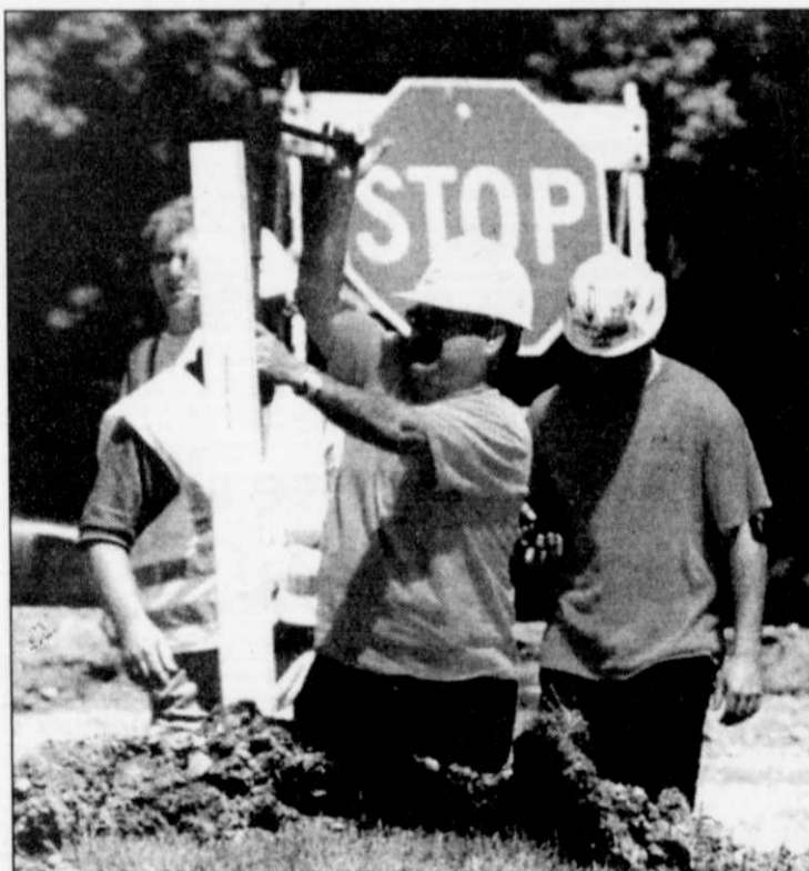
A worker from WE Energies shuts off the gas main at Timblin Drive and USH 45 after a gas line was ruptured.
