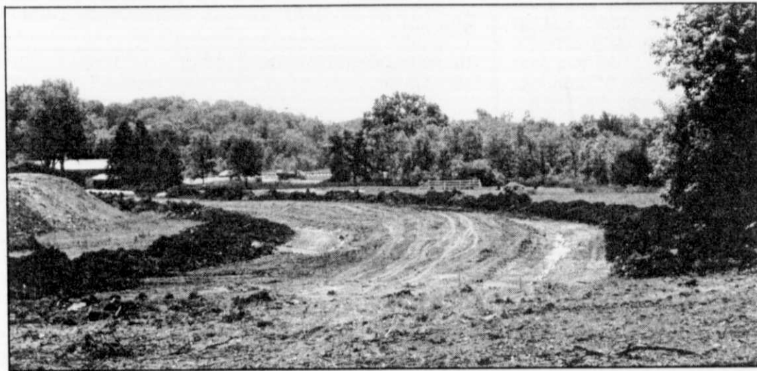
Shown above is a view of the grading for the new Badger Road that is being constructed.
