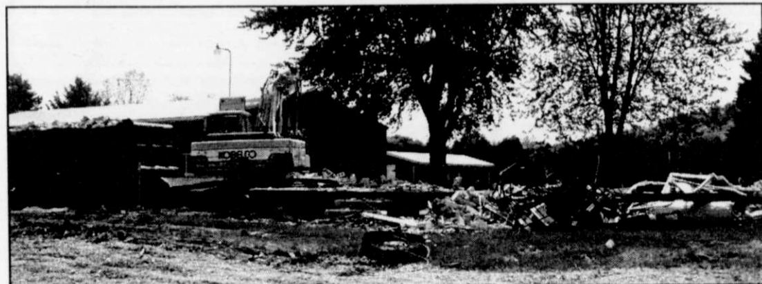
Crews from Badger Wrecking in West Bend work on removing the home of Maurice Struebing. The home was sold to the state to make way for an improved USH 45 CTH H east Badger Road intersection. Statesman Photo: Andrew Kuehl
