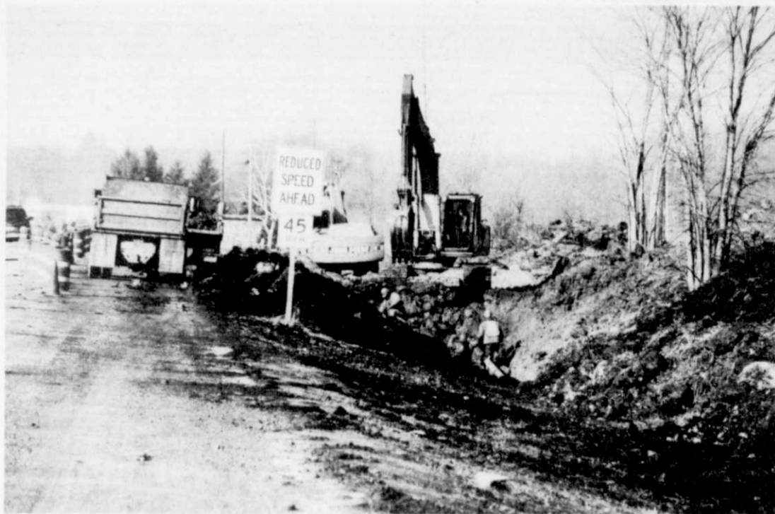
Shown above are workers from WE Energies lowering a gas main to make way for the new roadbed.
