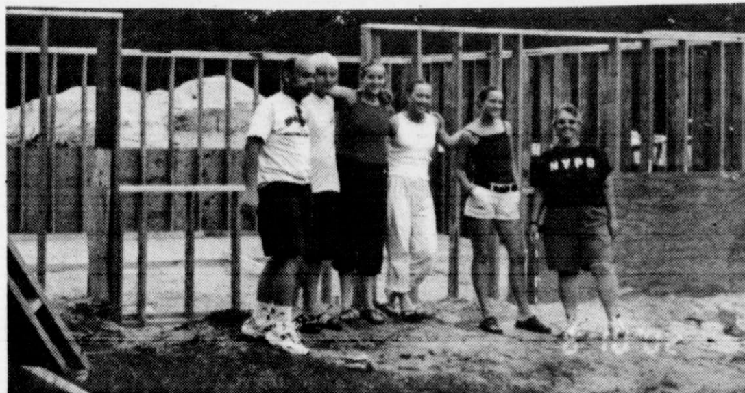
Left to right: Dan Runquist, Brandon Gitter, Stacey Imler, Emily Ogi, Jamie Imler, and Sheri Rehn in front of the house frame.
