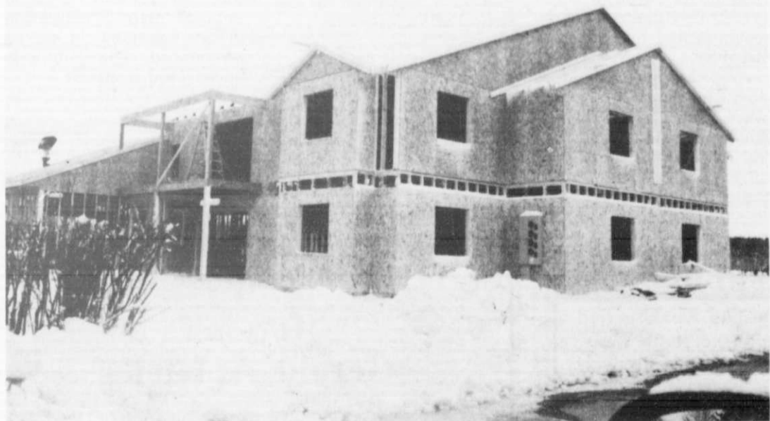
The first of Kewaskum's newest condos are well underway. The condos, being developed by Emmer Real Estate Group, are being built off of Roseland Drive in Kewaskum. The first condos are expected to be completed this spring.
