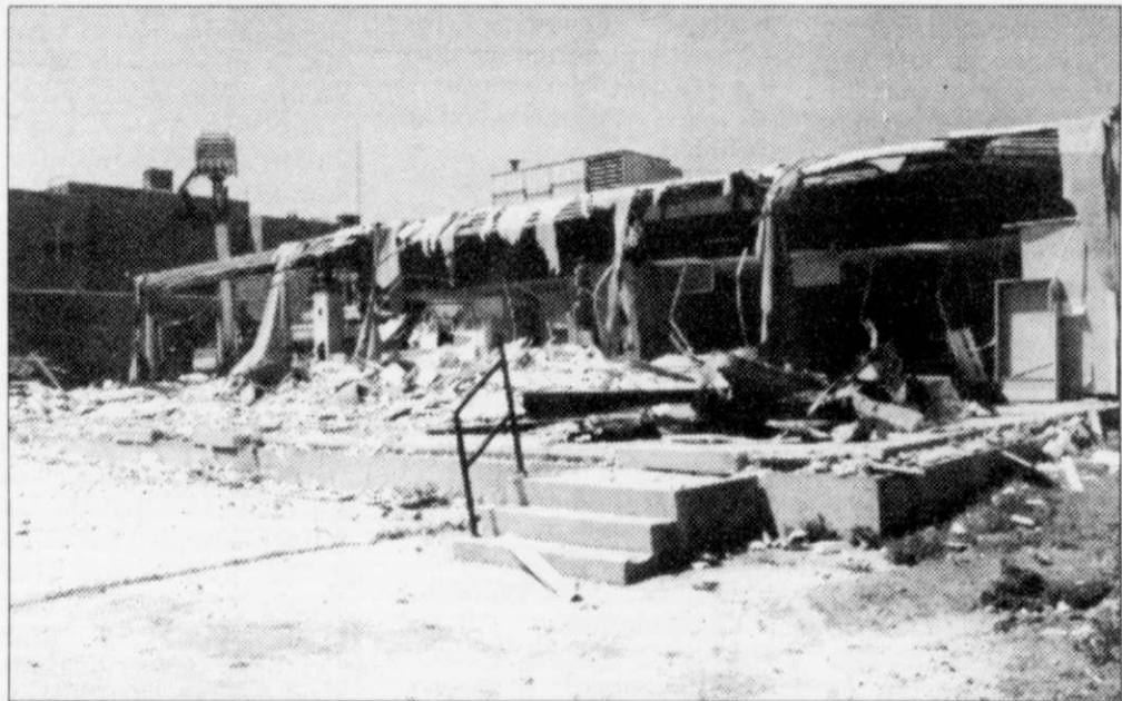
Demolition of the old Kewaskum Elementary School began Monday. Crews started in the back of the school and by press time the library and classrooms in the vicinity were completely razed. Statesman Photo: Andrew Kuehl
