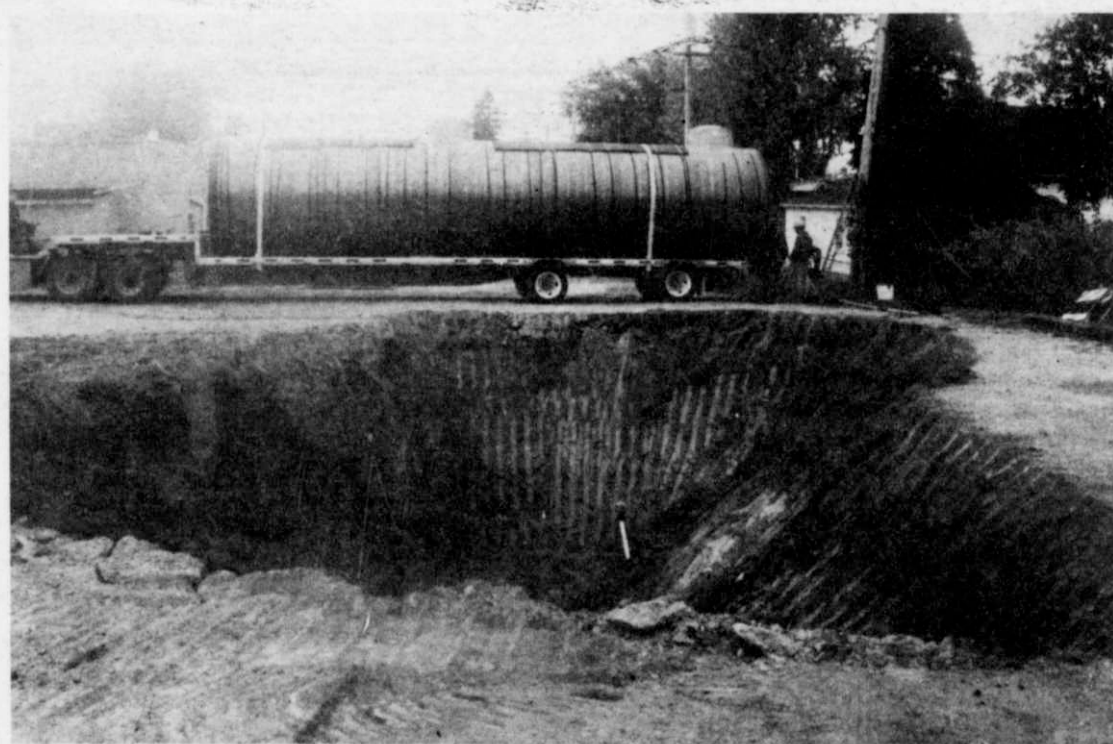
A photo showing the 20,000 gallon tank about to be installed and the hole it will be buried in.
