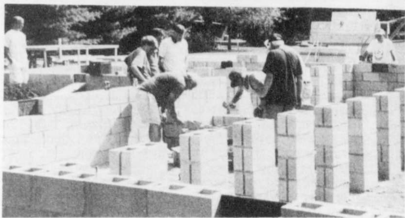
The first two days' efforts lay a solid foundation for the wooden structure to come.
