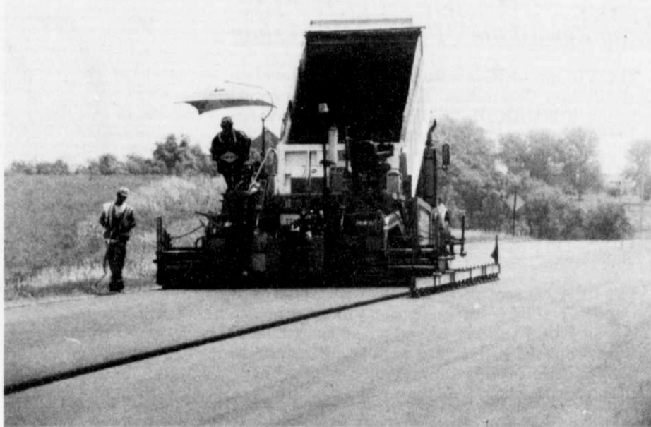
Paving on CTH H west in the Town of Wayne continues. The project is being funded by the Washington County Highway Commission using general transportation aids and Local Road Improvement Program funds from Wisconsin D.O.T.. The work west of Wayne is being done by Payne and Dolan. Work east of Wayne is being done by Scott Construction.
