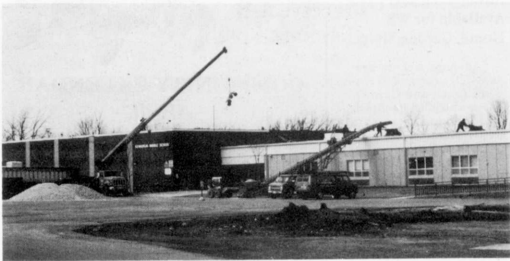
Repairs to the existing roof at Kewaskum Middle School were begun in the evening late last week by J. T. Roofing of Newburg. The repairs were expected to be completed this week while students were enjoying their spring break and all should be back to normal by the time school is back in session on Monday. (Statesman photo: Andrew R. Kuehl)
