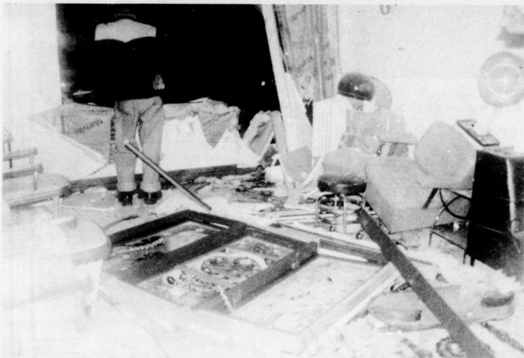
This photo displays just some of the massive destruction the interior of the building incurred following the impact.
