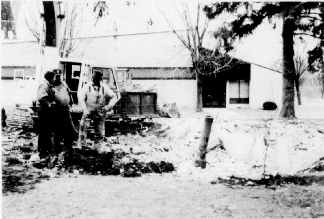
The rental building owned by the Village of Kewaskum, located at 1102 Fond du Lac Avenue, adjacent to the Kewaskum Fire House was razed on Wednesday, December 28. After much discussion, the Village Board voted unanimously to raze the property at their November 7 board meeting. Shown working on the hole left after the building was taken down is Director of Public Works Jerry Gilles, left, and Village Employees Alan Kuehl, center, and Craig Gruber, right.
