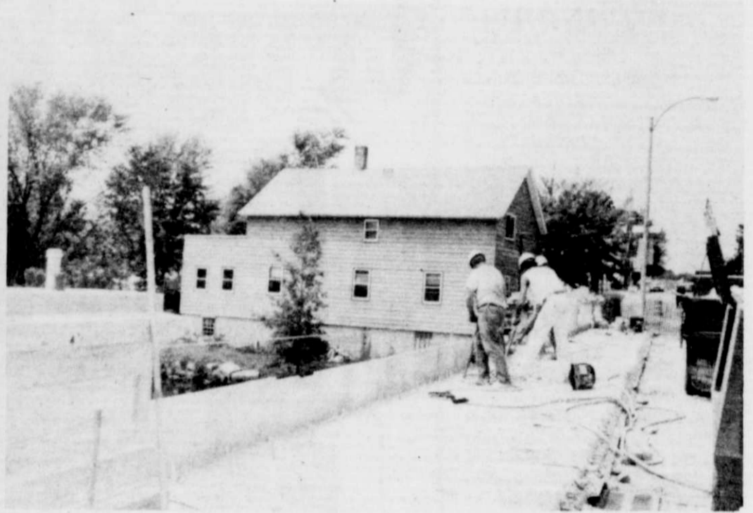
Repair crews removed the concrete railings, sidewalks and roadbed of the bridge.
