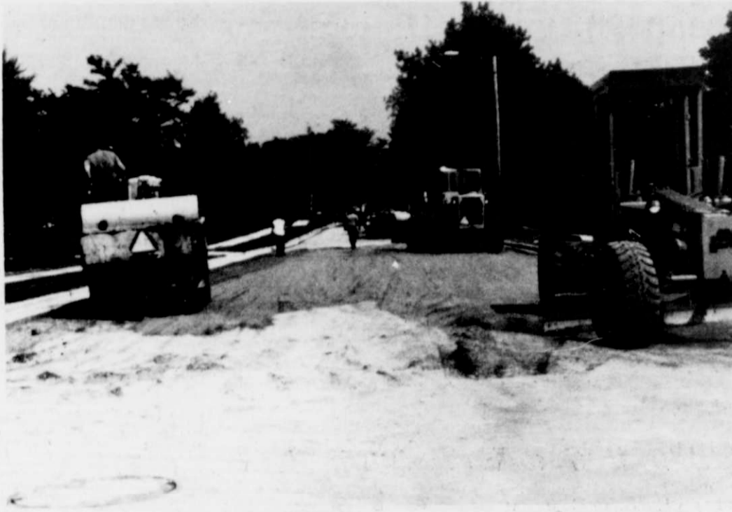
Work has been completed on the street in front of the Dr. Cesar Sison home on Forest Avenue to the intersection of Edgewood Road in Kewaskum. The old blacktop was removed due to breakup causes. The blacktop was dug up and the underneath substance of wet marsh clay was also removed. It was then filled with gravel and repaved. Payne and Dolan was the contractor.
