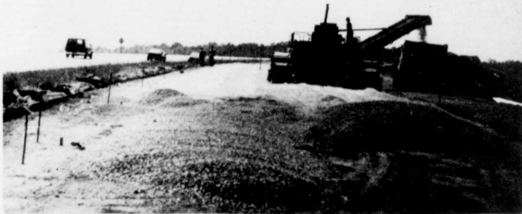
Machinery spread gravel in preparation for laying concrete along a portion of the final two lanes of the Highway 45 bypass.
