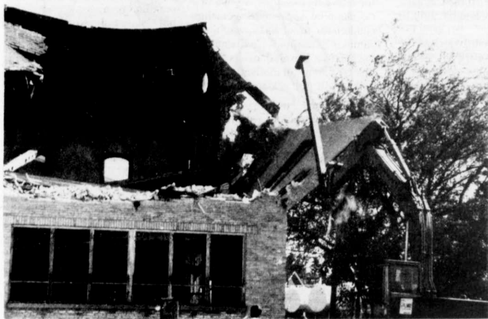
The second story portion of the school's west wall crashed to the ground as the steel wrecking arm continued to pick away at the building.
