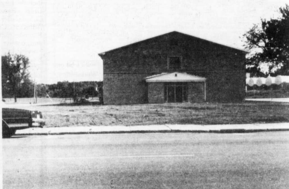
With the demolition of its predecessor complete, Holy Trinity's grade school is now visible from Main Street.
