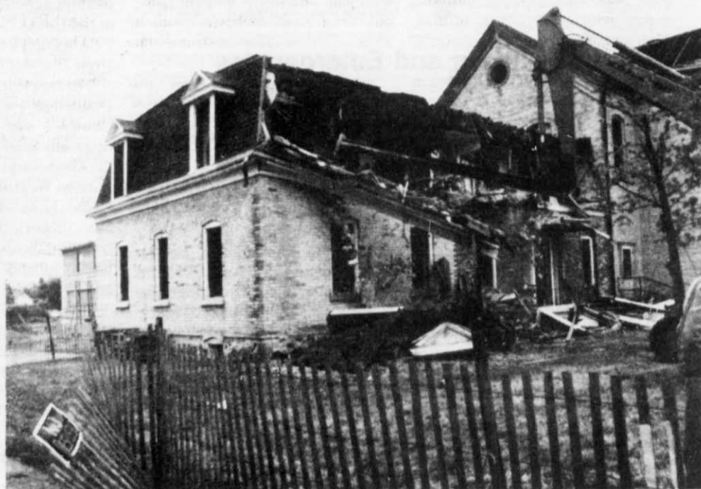
The front section of the convent wall fell exposing rooms which had been home to nuns which had staffed the school for 98 years.
