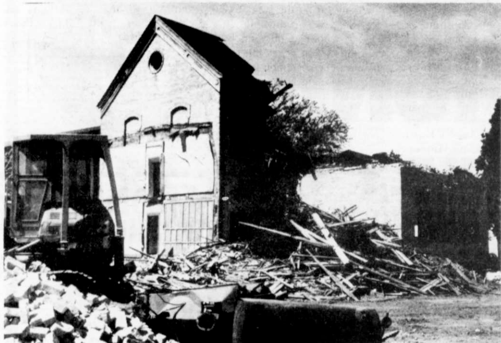
Piles of brick and rubble were soon all that was left of the convent and school which had withstood wind and weather for over 100 years.
