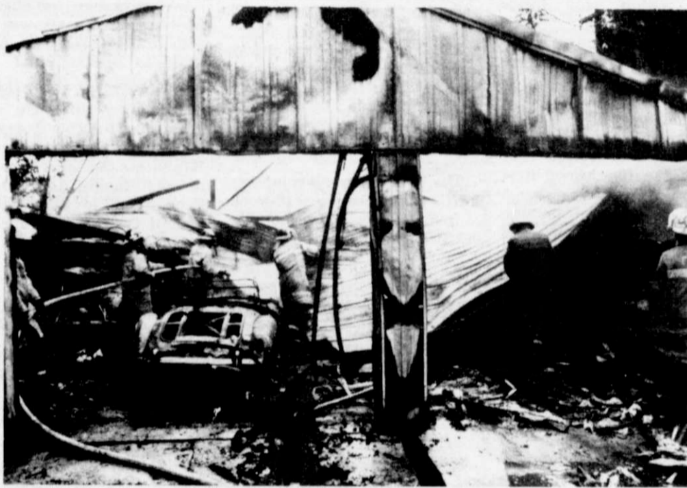
Kewaskum and Campbellsport firefighters extinguished flames in the Geidel garage. Also destroyed were two antique cars stored in the structure.
