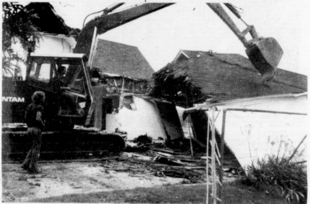
One big bite of the shovel and the garage of the former Weddig property is a pile of broken lumber and shingles. Statesman Photos by Gerry Mueller
