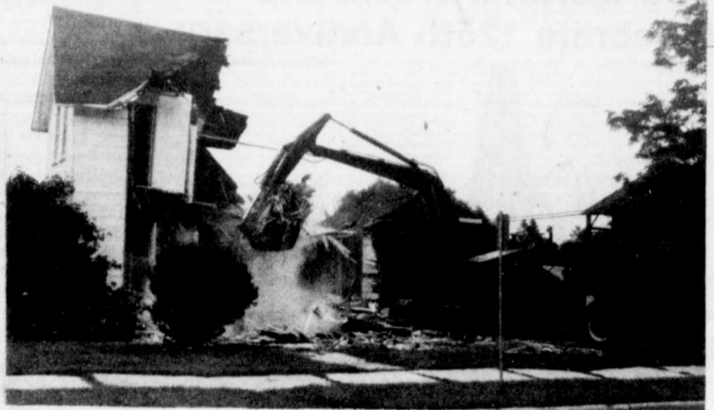
THE FORMER ROSE WEDDIG HOME, 1404 Park View Drive, was reduced to rubble by a wrecking crew last week. The property was purchased last year by the St. Lucas Church, which plans to use the land for future expansion of its Christian Day School directly north of the property.
