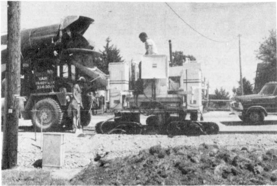
A cement truck pours concrete into the hopper of the "Vari-Former" which automatically lays a continuous ribbon of cement creating a sidewalk without the need for any steel forms being laid.
