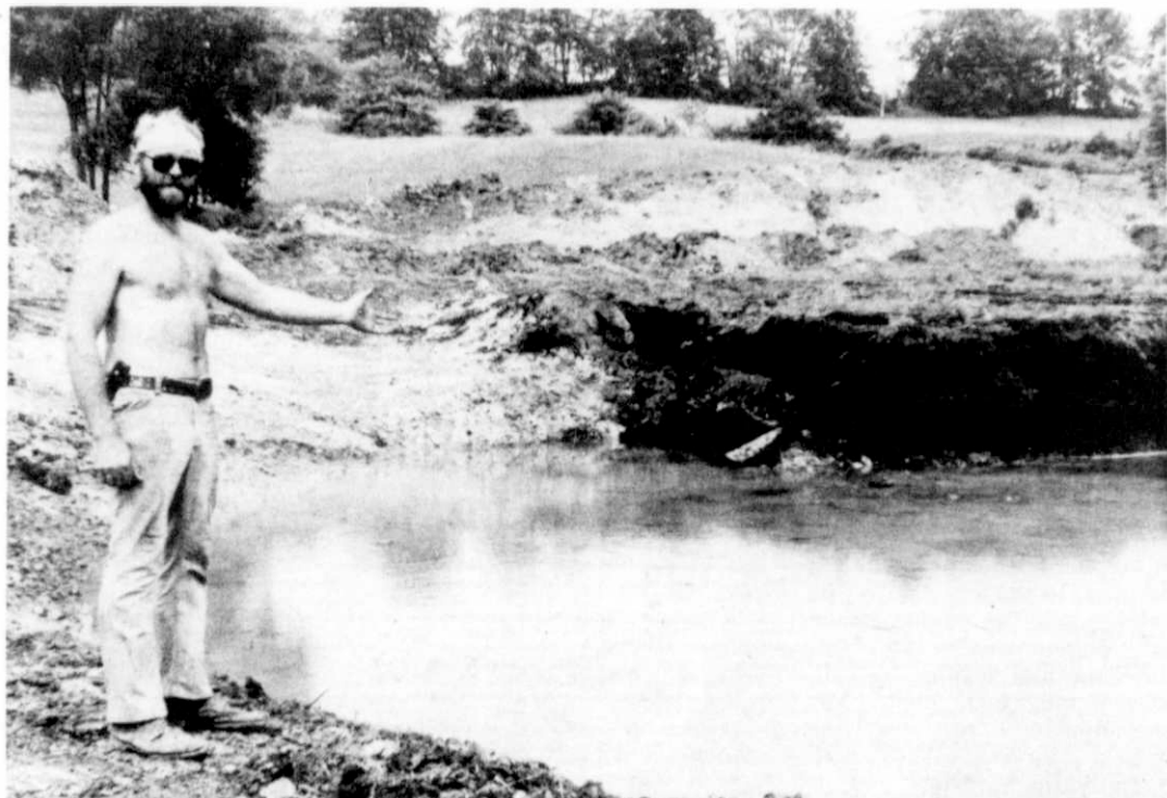
SUNBURST SKI HILL Mgr. Gary Ciriacks and the new ten million gallon plus pond now under construction at Sunburst. They are also burying 3000 ft. of new pipe for increased snow making capabilities. Five large Snow Cannon snow making machines are being added for the 1985-86 ski season. A second chair lift is in their long range planning. (Chuck Voge photo)
