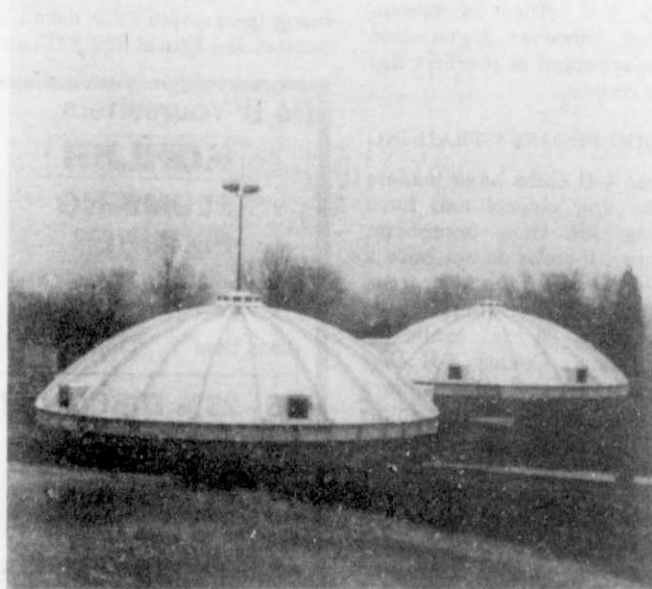
Kewaskum's new Clarifier Covers at the Sewage Treatment Plant.
