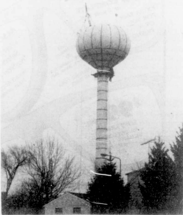
The sphere is complete except for the top panels which were expected to go in place this week.
