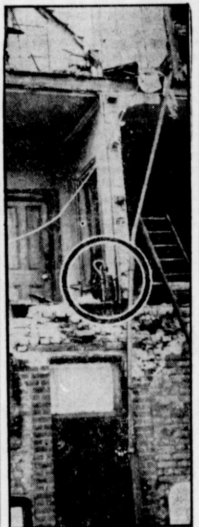
WRONG PROTECTION—Prudent owners of this house in West London, England, have kept their portable air-raid warden pump (circled) ready for use all these years, but they never dreamed a freak wind-storm would slice off the side of their dwelling. No one was injured by the strange "twister" of fate.
