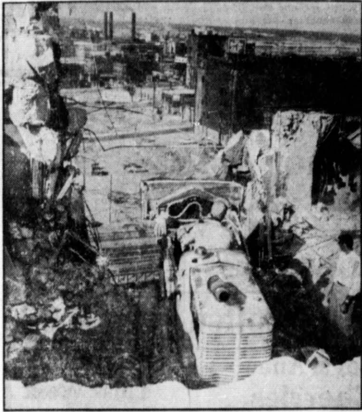
NO DOZING ON THIS JOB —It takes a wide-awake operator to "dig" a bulldozer through an 11-story building from the roof to the basement. The 19,000-pound machine was assembled atop a building being wrecked in Kansas City, Mo., and used to push debris over the side of the structure as it was demolished, floor by floor.
