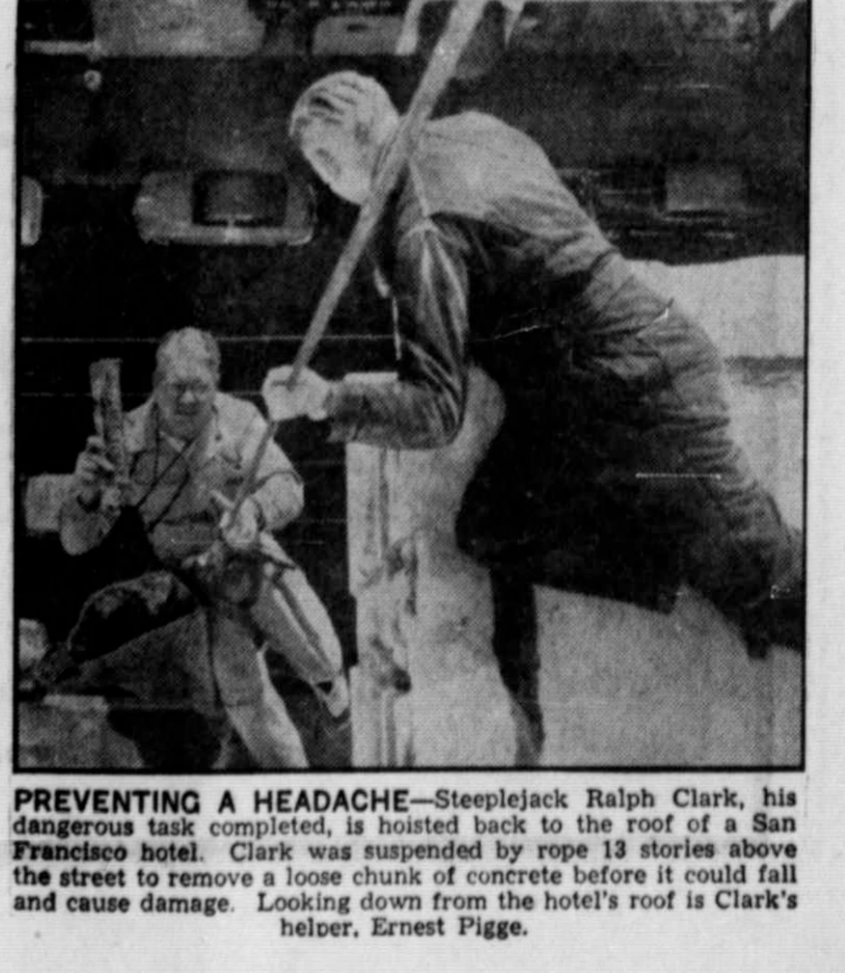
PREVENTING A HEADACHE —Steeplejack Ralph Clark, his dangerous task completed, is hoisted back to the roof of a San Francisco hotel. Clark was suspended by rope 13 stories above the street to remove a loose chunk of concrete before it could fall and cause damage. Looking down from the hotel's roof is Clark's helper, Ernest Pigge.
