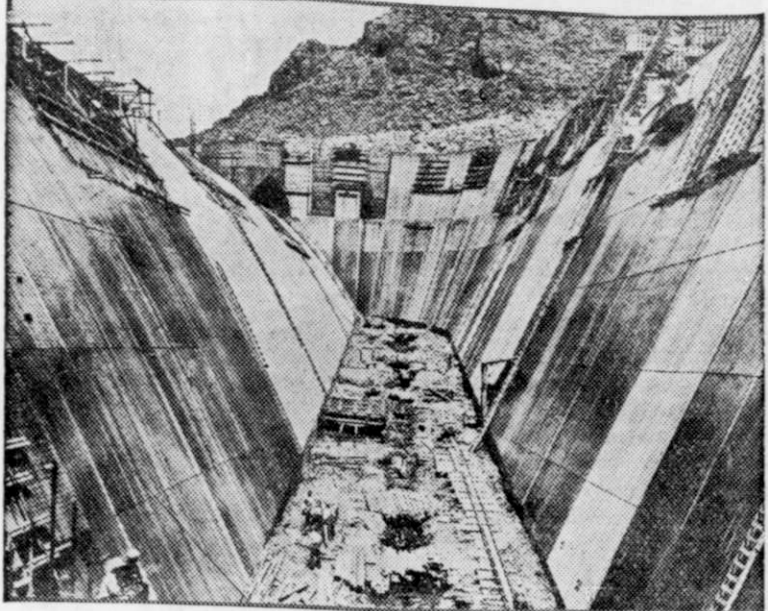
View upstream showing the nearly completed Arizona spillway of Boulder dam, through which the Colorado river will be diverted.
