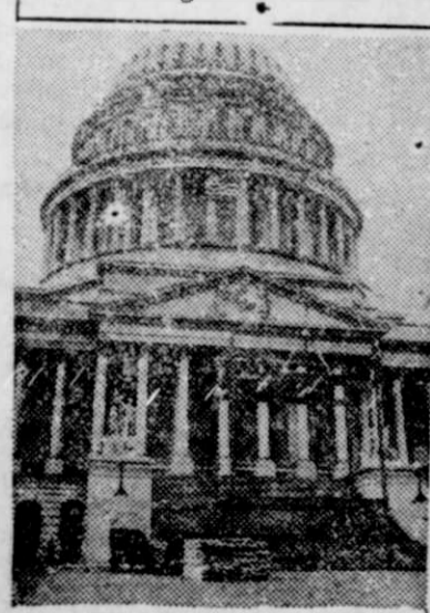
The partially completed inaugural stand in front of the Capitol where Herbert C. Hoover will take the oath of office as the thirty-first president of the United States.
