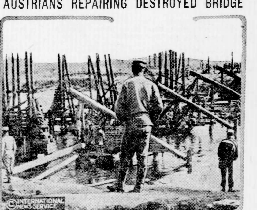
This photograph, taken during the retreat of the Russians through Galicia, shows Austrian troops repairing bridges.
